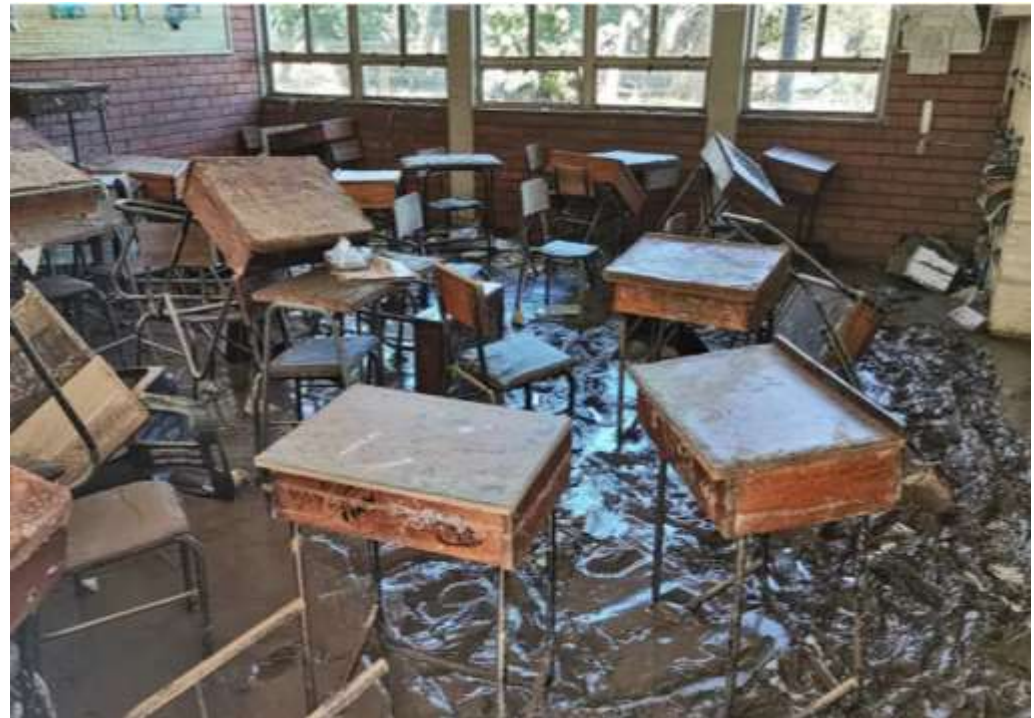
A mud-filled classroom in eThekweni, KwaZulu-Natal caused by unprecedented high rainfall and flooding on 11 April 2022.
